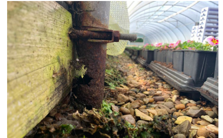
Non-ArmourGuard Corroded Ground Tube
