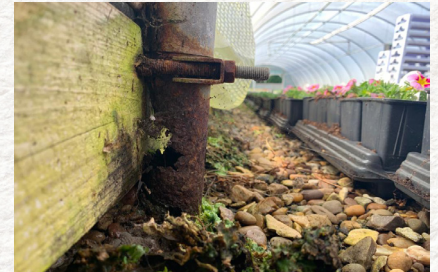
Non-ArmourGuard Corroded Ground Tube
